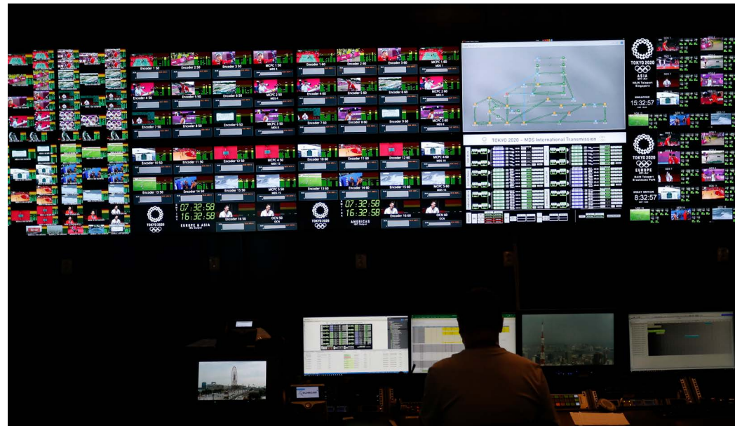
© 2021 Olympic Broadcasting Services / Silvio Avila The International Transmission room in OBS Tech ensures worldwide delivery of the signals to the RHBs' home territories.
